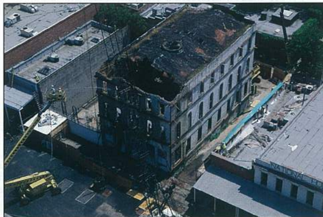
Demolition of the Tuesday Club yielded 84 tons of metals and 1,000 tons of concrete and masonry in addition to 314 tons of wood.
